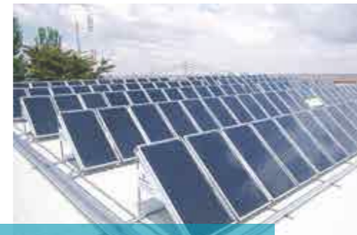
Solar thermal panels with automatic, differential temperature control systems to rationalise energy input and efficiency.
