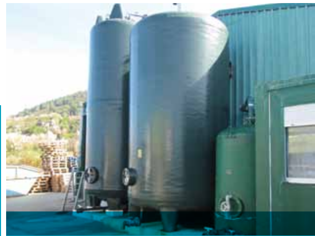
Secondary tanks for degassing and bubble removal, water treatment before its distribution to plant
